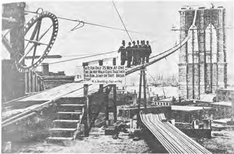
14 J. A. and W.A. Roebling, Brooklyn Bridge, New York, under construction, c.1877. Initial cable-spinning in progress.
